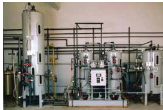
Portable Exchange Deionizer Regeneration Plant
